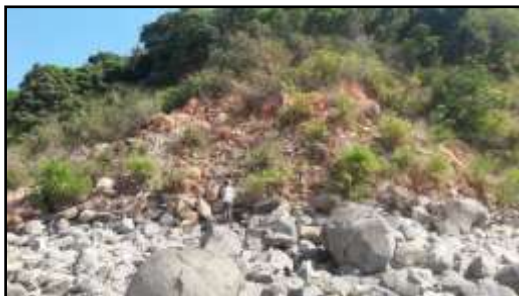
Figure 9. Landslides and rock fall causes by unstable slope fail of coastal sea-cliff
