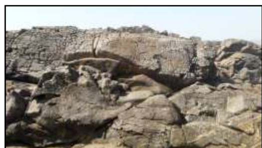
Figure 6. Development and subsequent widening of capillaries and larger cracks on the rock surface by weathering
